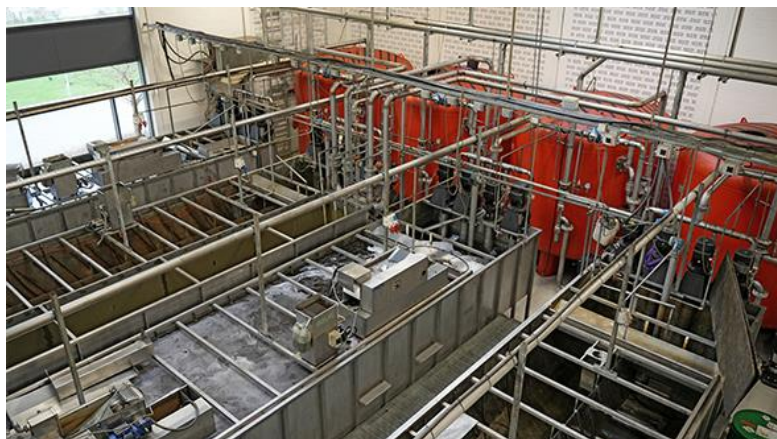
Kyocera Unimerco coolant plant in Sunds, Denmark
